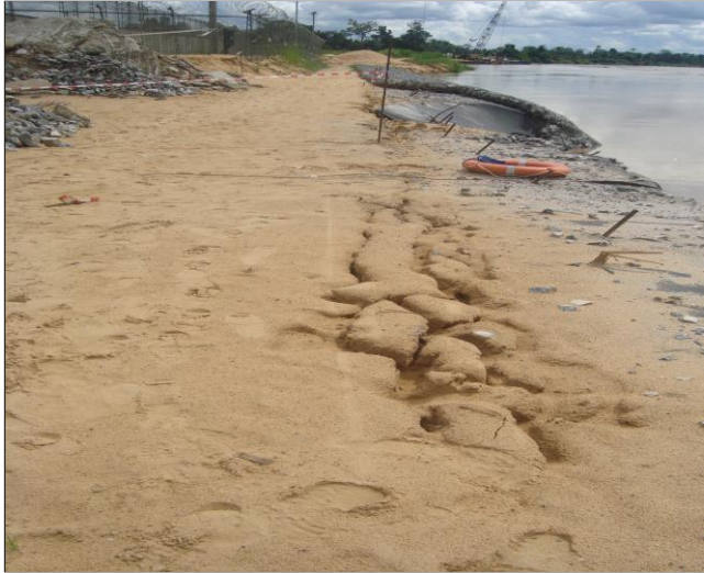
Figure: 35b Cracks observed on the ground at the onset of failure
