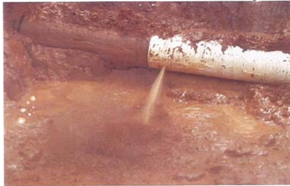
Fig 7.4: A section of a high pressure oil pipeline in Umuechem Community of Etche Local Government Area of Rivers State, Nigeria, showing a point of crude oil leakage (Wegwu and Omeodu, 2010)
