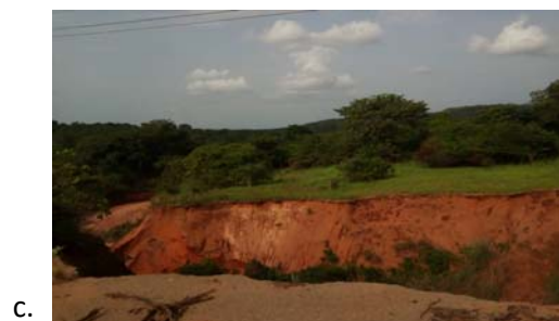
Figures 7.22a, b and c: Impact of gully erosion in Isuikwuato LGA of Abia State 7.2.3 Majoring in the Minor: The bane of Nigeria's geosphere.
